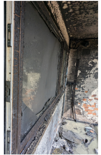
Fire damage to balcony
